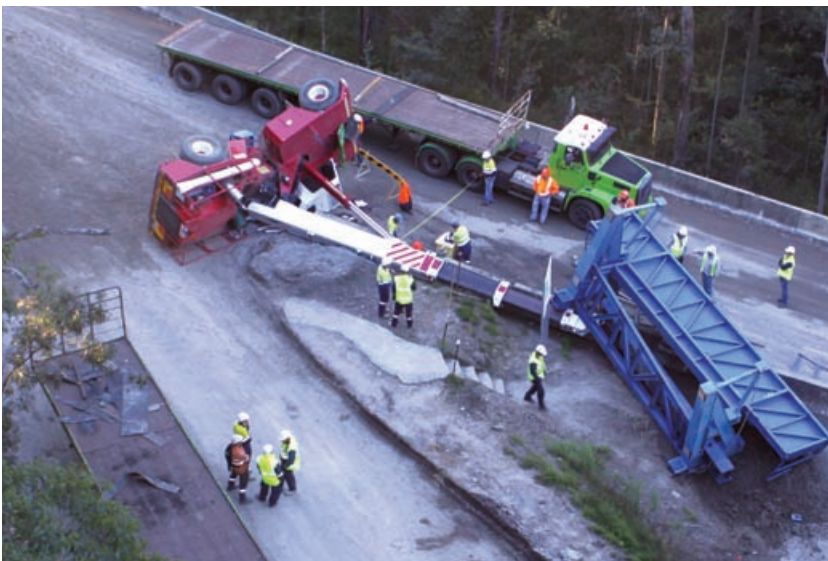
Image of tipped over crane
